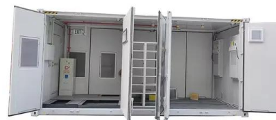
1075KW HH ESS
