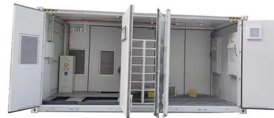
1075KW HH ESS
