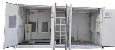
1075KW HH ESS
