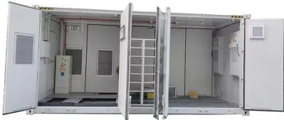
1075KW HH ESS
