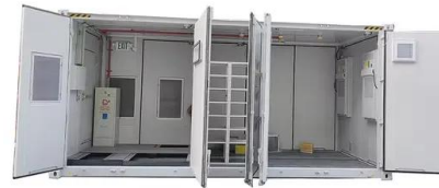
1075KW HH ESS
